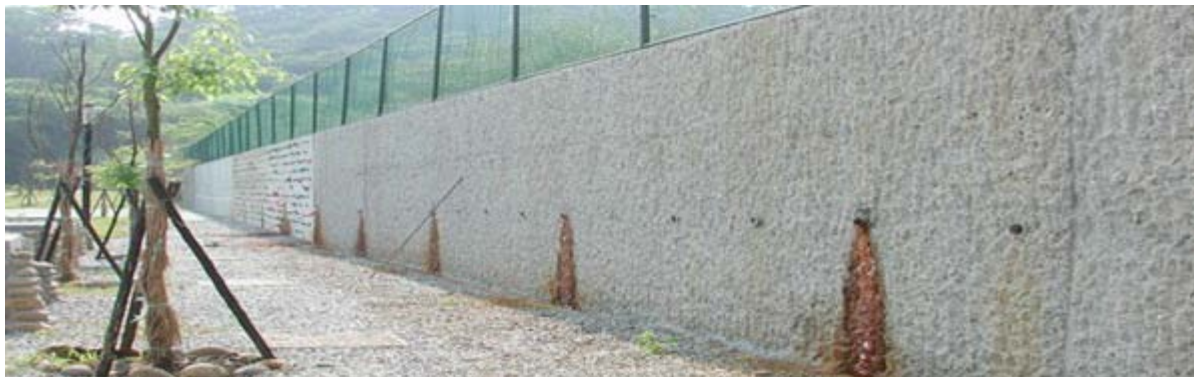
DRAINAGE BLOCKED FROM MINERAL SLUDGE EXCEPT WATERBELT OUTLETS
