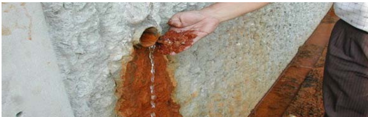
DRAINAGE CONTINUES DESPITE SLUDGE
